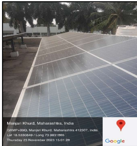
Photograph of Roof Top Solar PV Plant:
